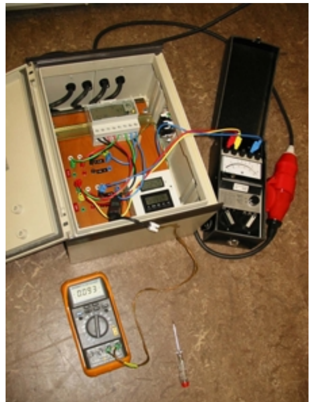
Fig. 3.2 Equipment for measuring standby consumption (EMU 32 3-phase, adaptable inputs/outputs, moving-coil wattmeter, sensor, multiple measurement device)
